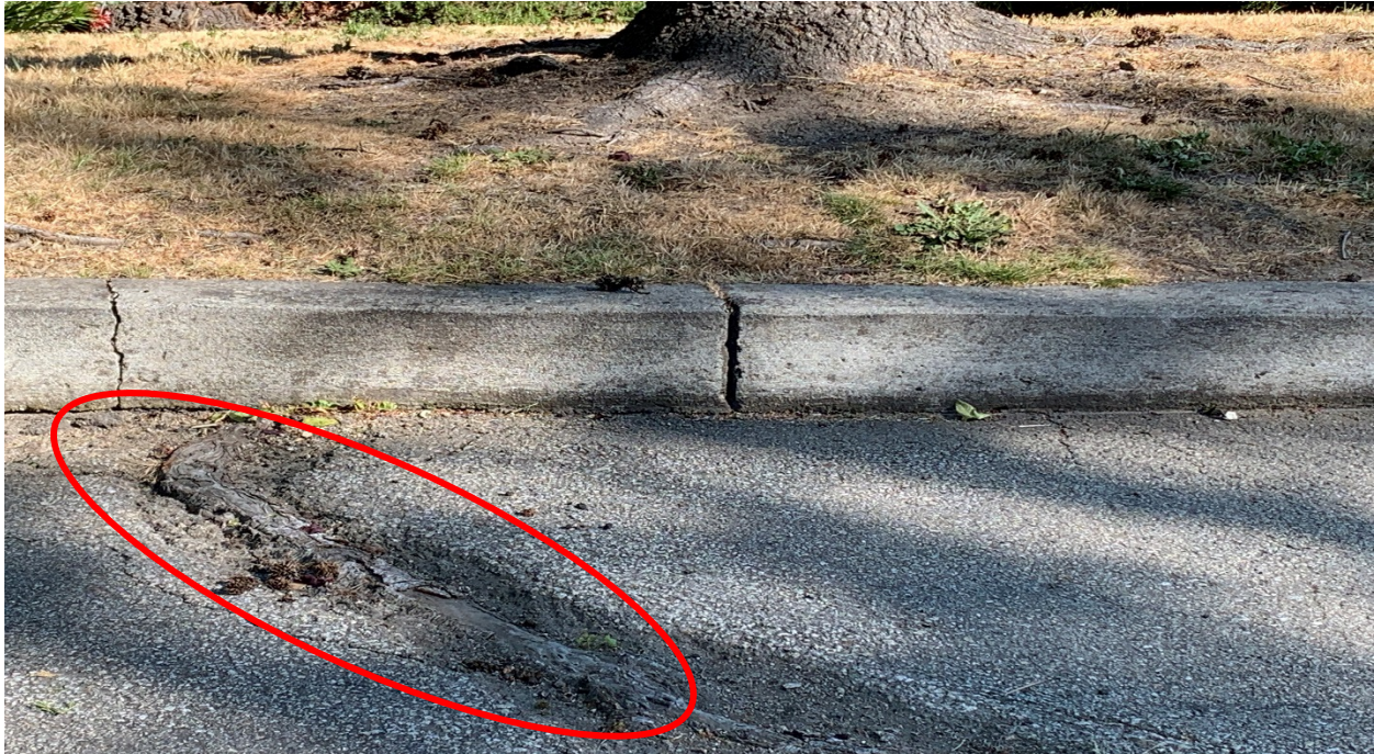
Image #4 – Tree T11, liquidambar. Note exposed root (circled).
