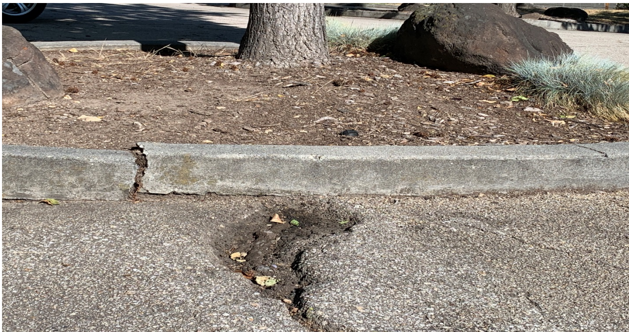
Image #5 – Tree T8, with exposed root in asphalt.
