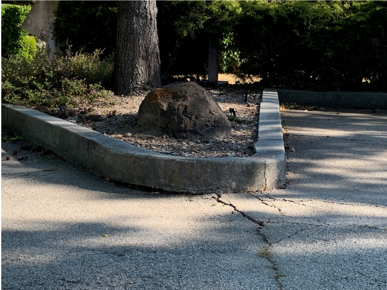
Image #3 – Tree T9, liquidambar. Curb and asphalt lifting and cracking.
