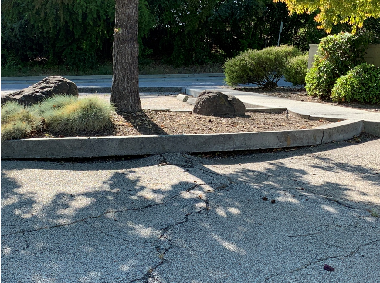
Image #2 - Tree T8, liquidambar. Note cracked and lifted curb and pavement.
