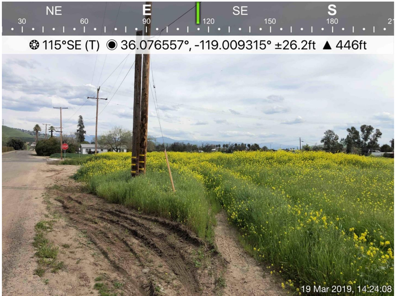
Photograph 20: Tire ruts along Grand Avenue right-of-way during site visit in March 2019.
