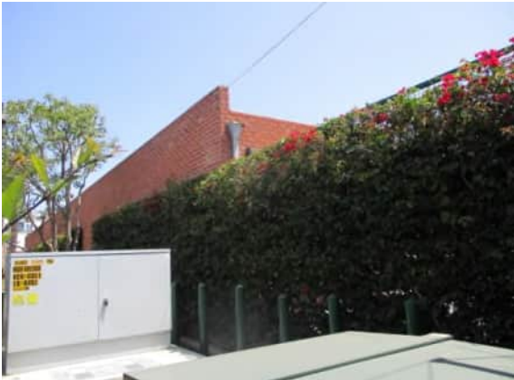
Photo #57: Pad mounted transformer
