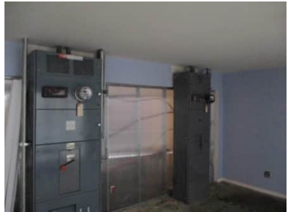
Photo #28: Main electrical
