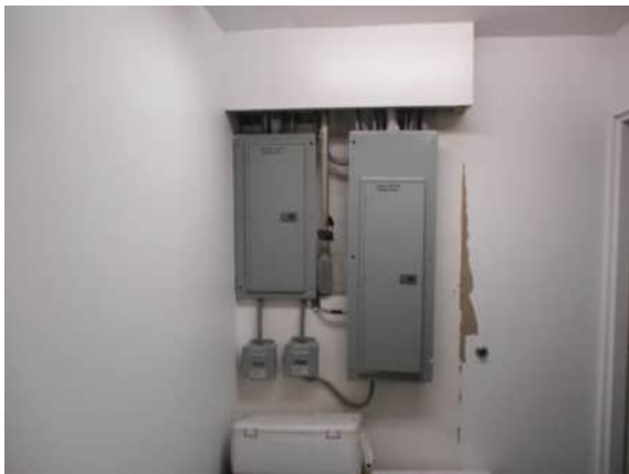
Photo #23: Electrical Panels
