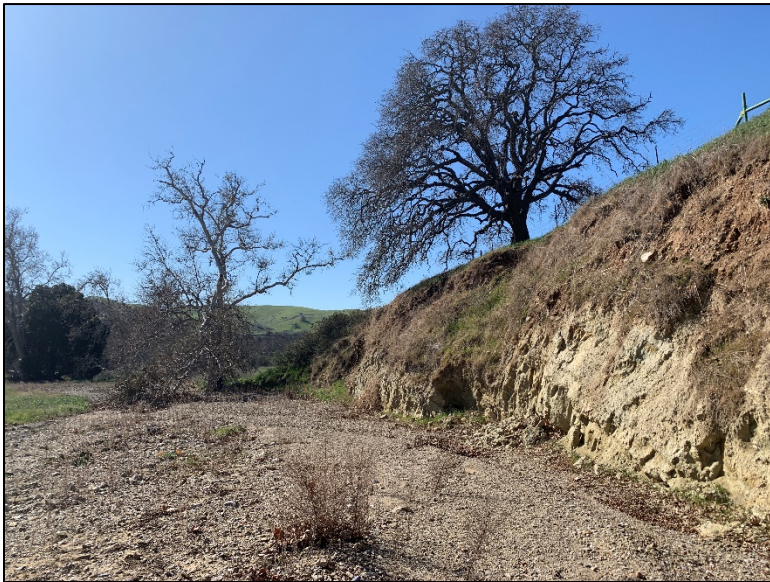
Photo 10: Representative photo of the riverine (ephemeral stream) habitat of Dry Creek located on the west side of the existing bridge, where the channel cuts into the bank of the riparian habitat area on top.
