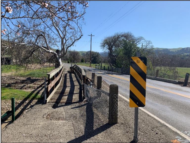
Photo 6: Photo of existing wooden pedestrian pathway on east side of bridge, looking south along Arroyo Road.
