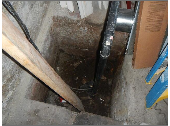
8. Sump in basement
