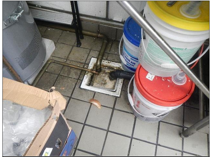
14. Floor sink or drain in tenant kitchens
