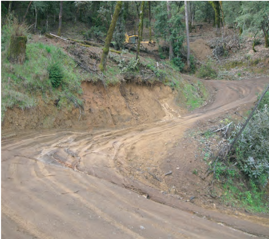
Photograph 3. Erosion on existing unpaved access road, 1111 Doolan Canyon Drive. Photograph by CGS, March 3, 2010.
