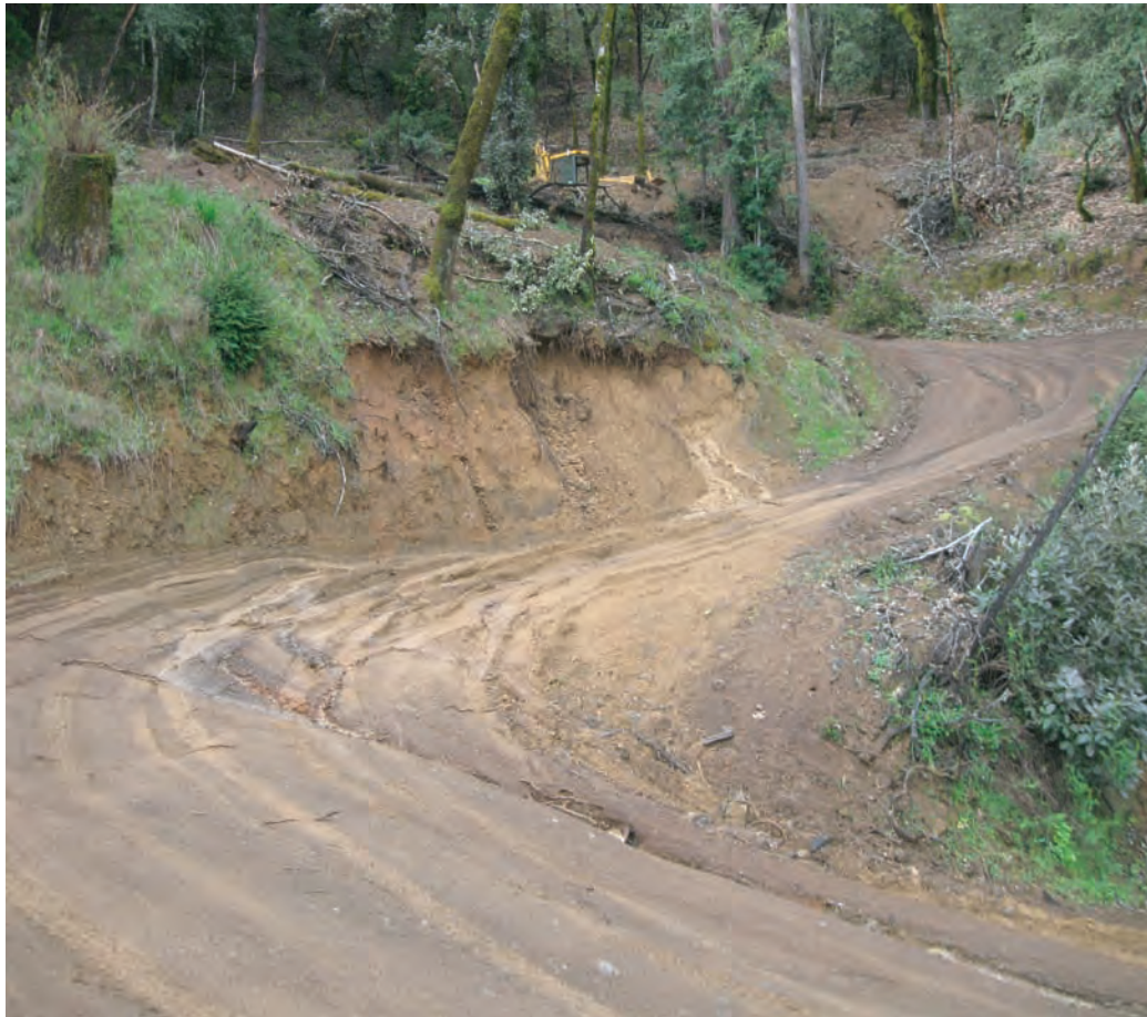
Photograph 3. Erosion on existing unpaved access road, 1111 Doolan Canyon Drive. Photograph by CGS, March 3, 2010.
