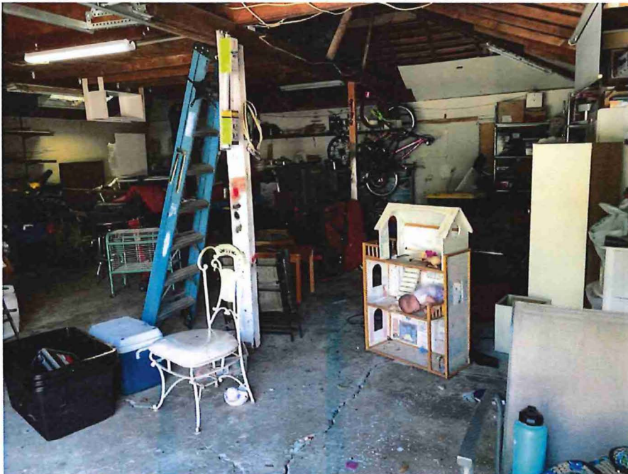
10. View inside garage, cracked concrete visible
