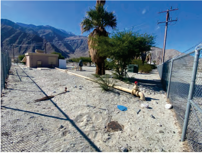
Photo 1: View from south side, looking southwest at existing Well #17.
