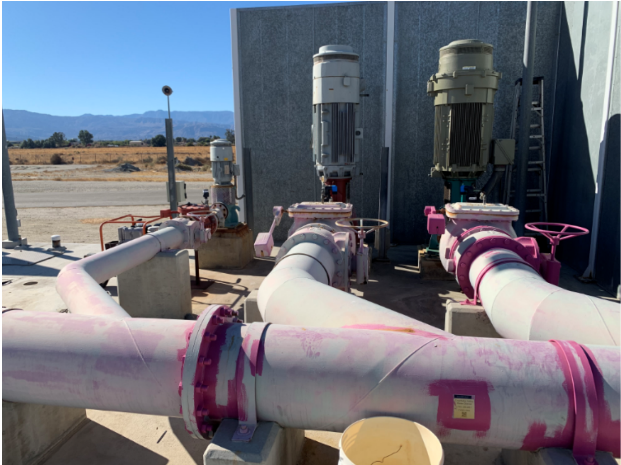
Figure 9: Existing NPW Pump Station
