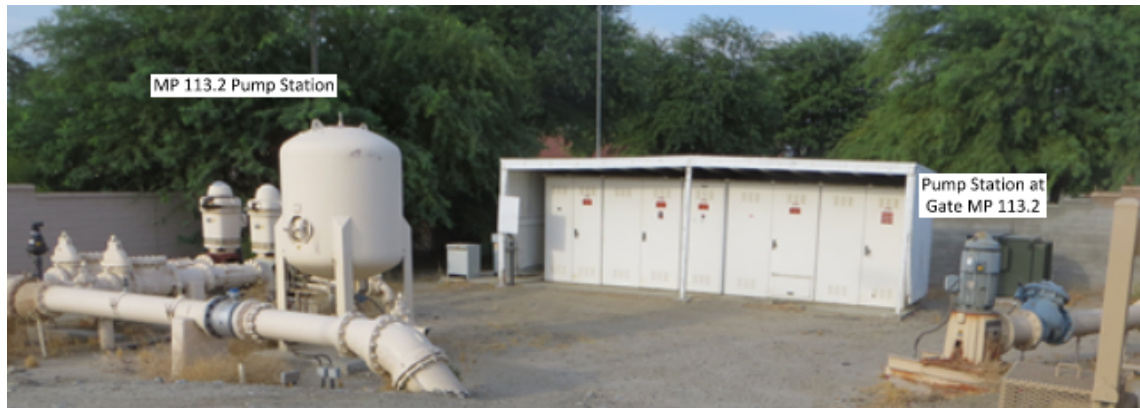
Figure 11: Existing MP 113.2 Pump Station (Left) and Pump Station at Gate MP 113.2 (Right)
