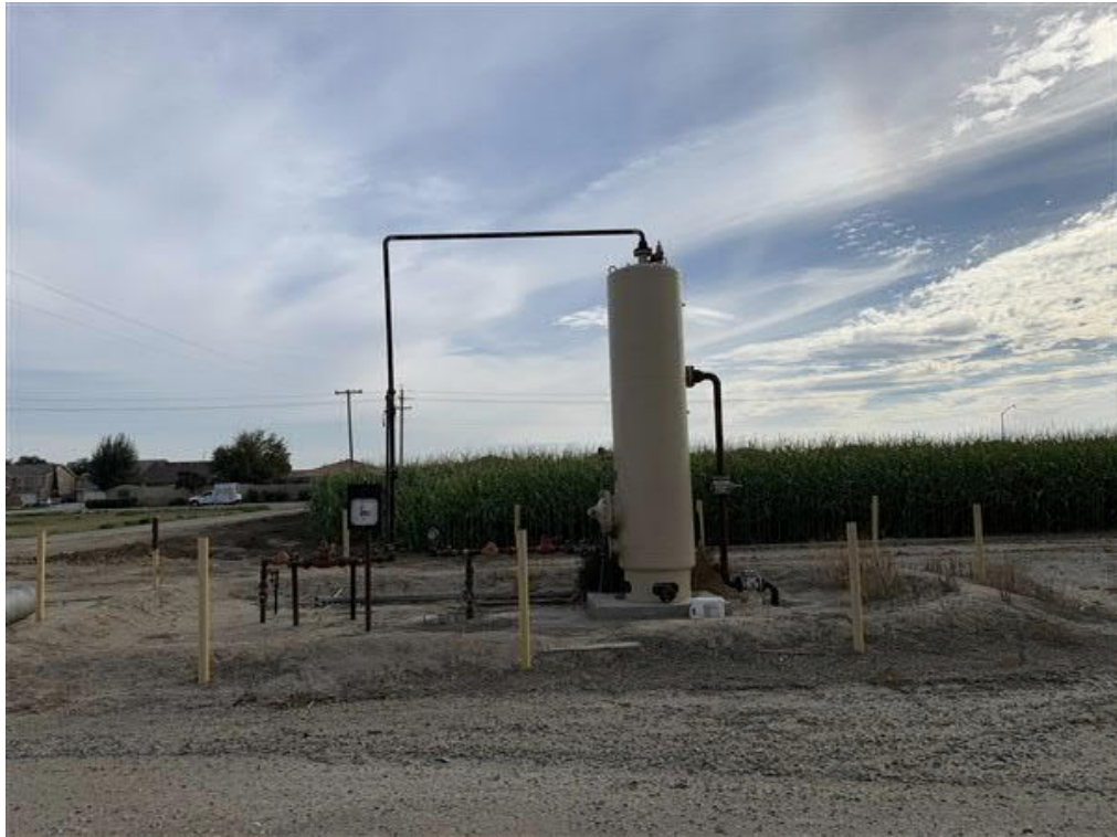
Photo 9: View of the gas separator apparatus that is located adjacent to the idle oil well 24A-24.
