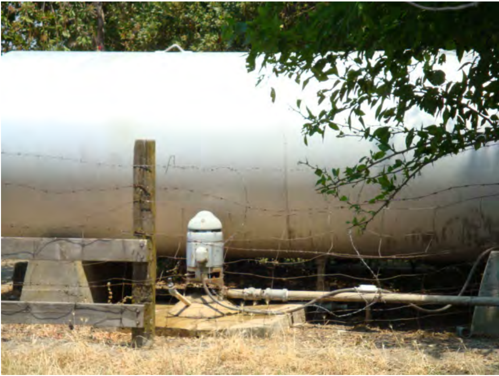
Photo 4 – Close-up image of pressure tank utilized by homes on Hess Lane.
