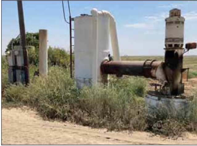
PHOTO 1: Irrigation pump discharging to irrigation canal
