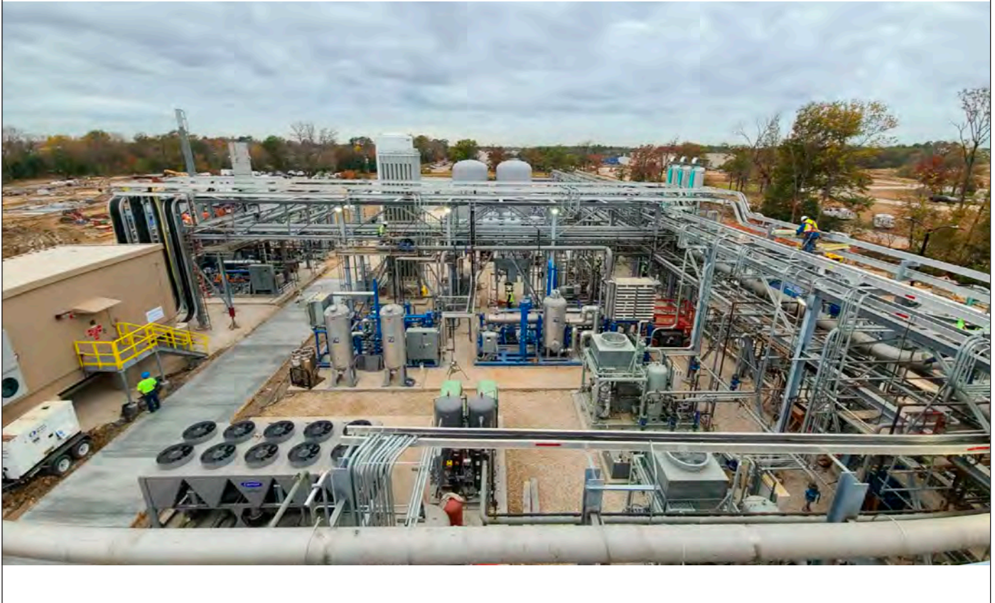
Figure 6 Typical RNG Plant
