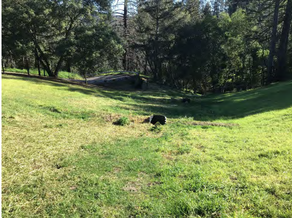
Photo 1 Drop inlet structure on the eastern portion of the site. Photo taken on March 22, 2022.
