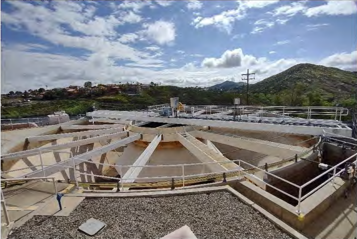
Plate 14. Up-flow clarifier, looking east.
