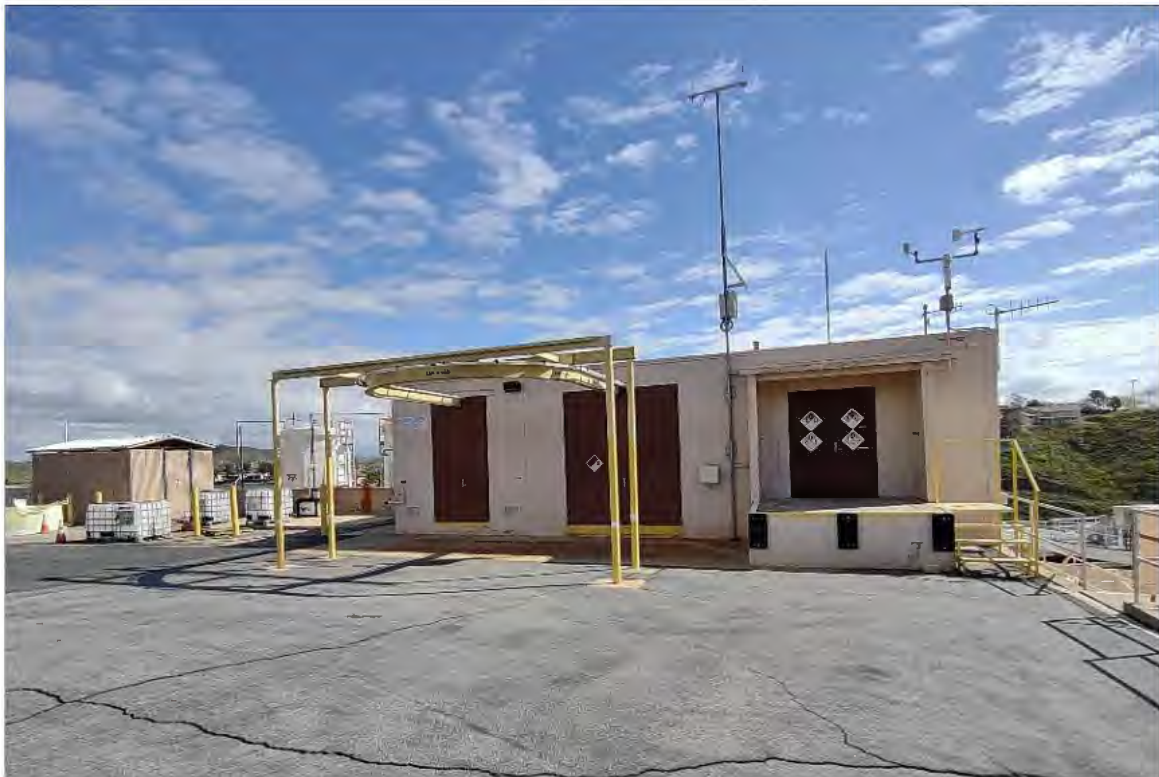
Plate 4. Chemical Feed Building 1 southwest façade with polymer storage pad and sulfuric storage enclosure at left, looking northeast.
