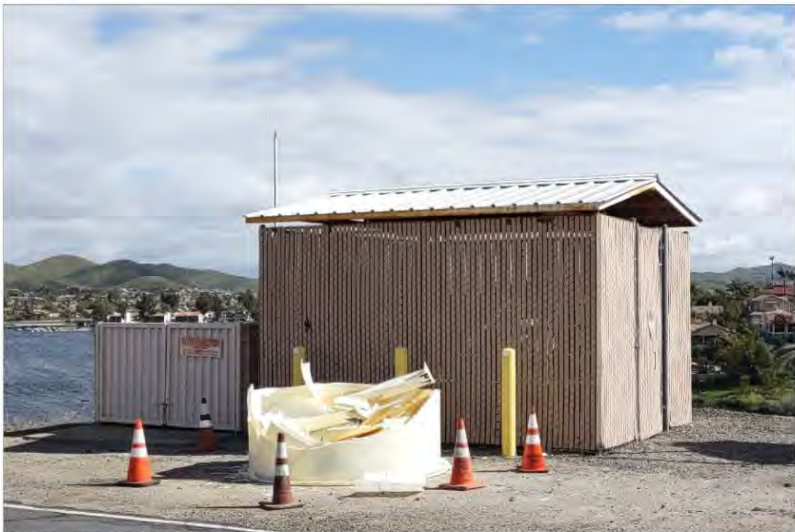
Plate 8. Chemical Feed Area 1 sulfuric acid roofed storage enclosure with trash enclosure to the left, looking northeast.
