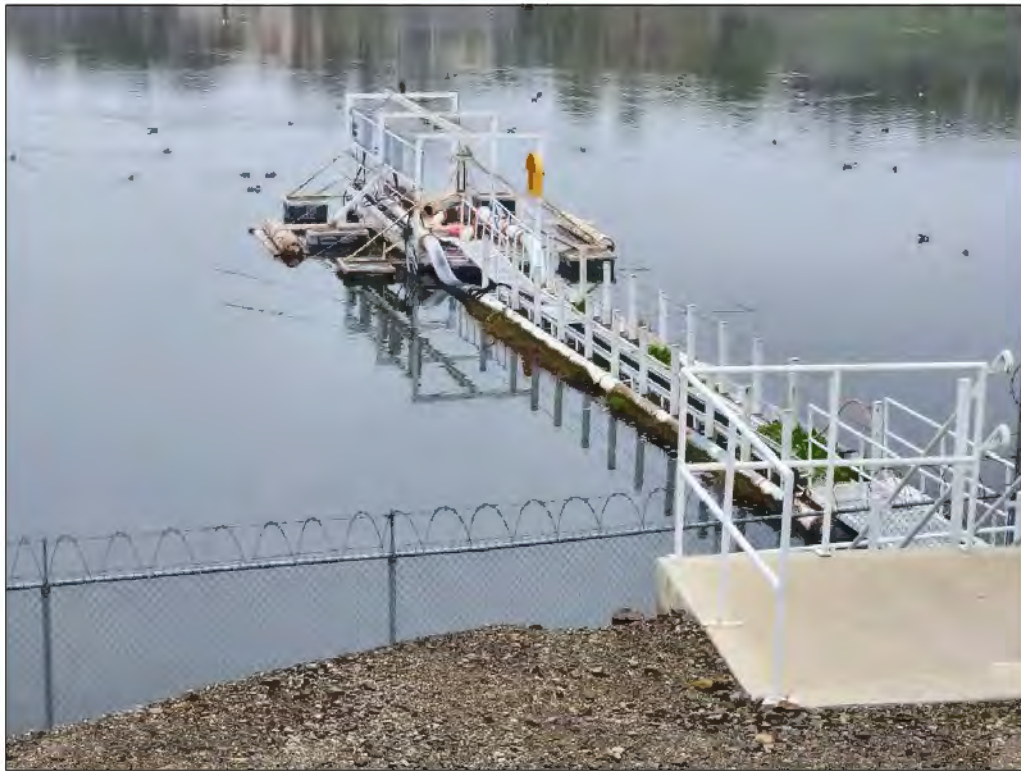
View looking north at dock to be removed and replaced. Photo taken March 17, 2023.
