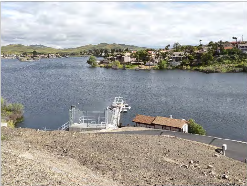
View of intake pump and barge with electrical building at right, looking north.
