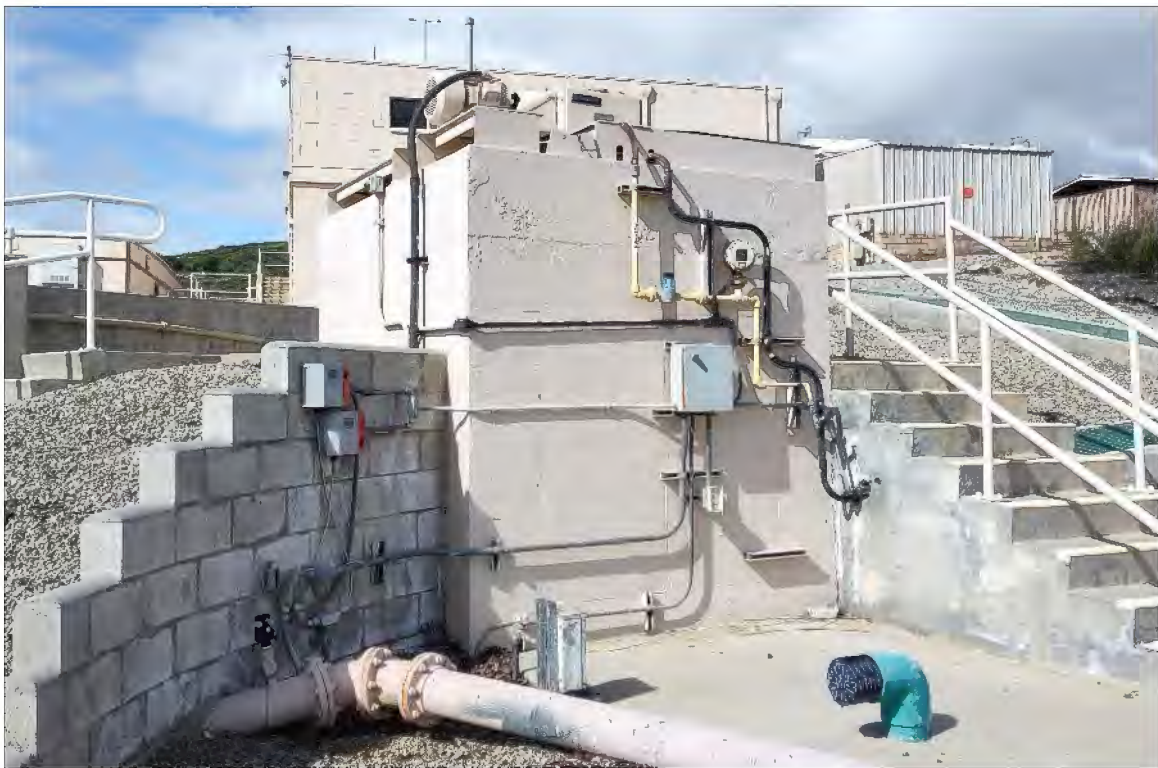
Plate 12. Rapid Mix enclosure, looking west.
