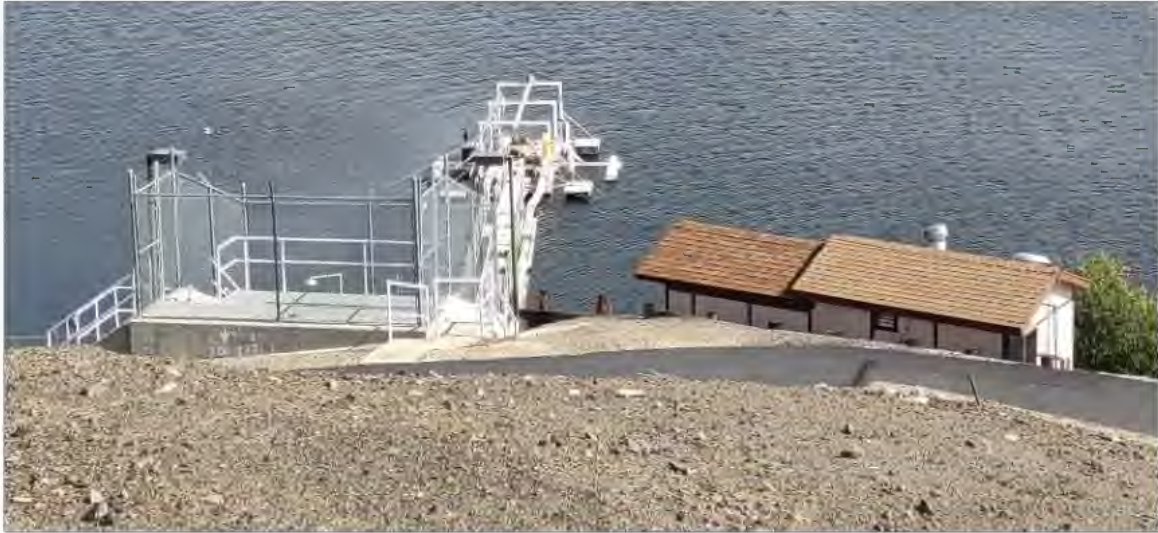
Plate 9. Intake pumps on barge, electrical building at right, looking north.
