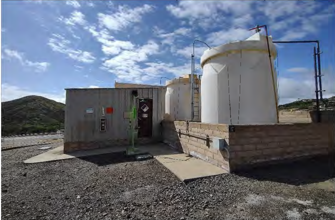
Plate 7. Chemical Feed Area 1 sodium hydroxide and ferric chloride storage tanks with slump stone containment wall at right, and sodium hydroxide storage building at left, looking south.
