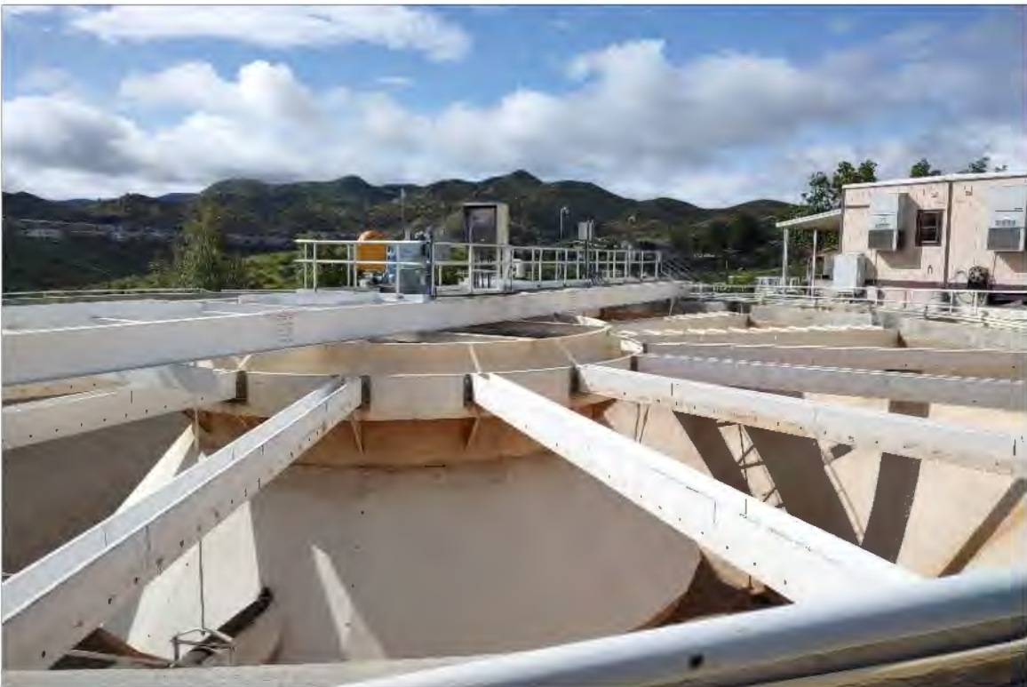
Plate 15. Detail of up-flow clarifier components, with operations building at right background, looking south.
