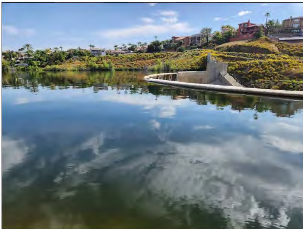
View looking north at spillway showing water level at spillway height. Photo taken May 16, 2023.
