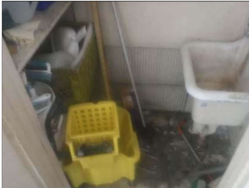
Photo 6: Janitorial Closet in Fellowship Hall Building
