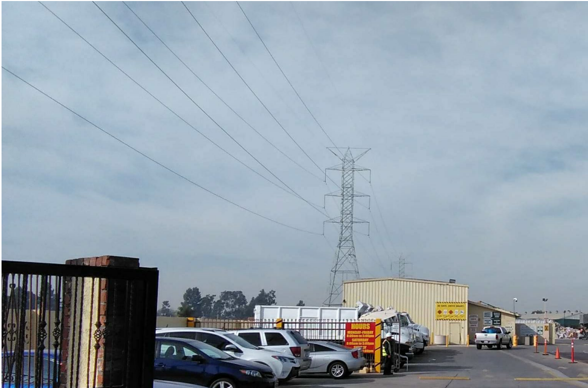
Figure 5-68. LADWP Boulder Lines 1 and 2, Taken near their Intersection with Rayo Avenue, West-Facing
