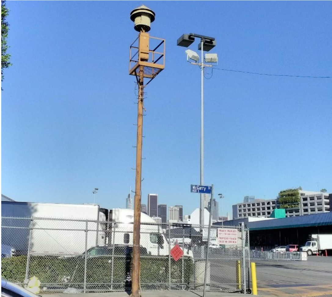
Figure 5-25. Air Raid Siren No. 189, Northwest-Facing
