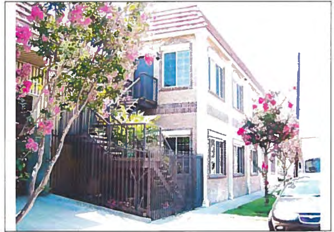
View looking southeast at metal staircase leading to second story entrance to 1991 addition.
