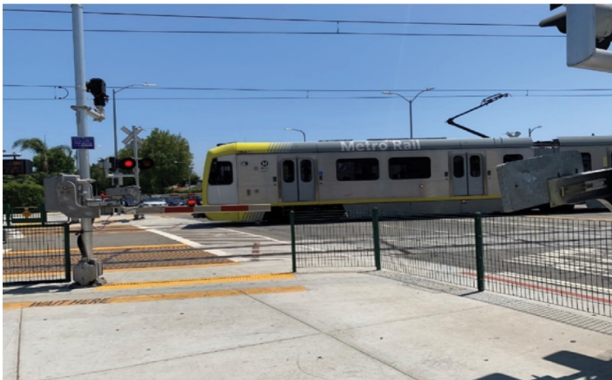
Pedestrian Gate Crossing Equipment on the Metro E Line
