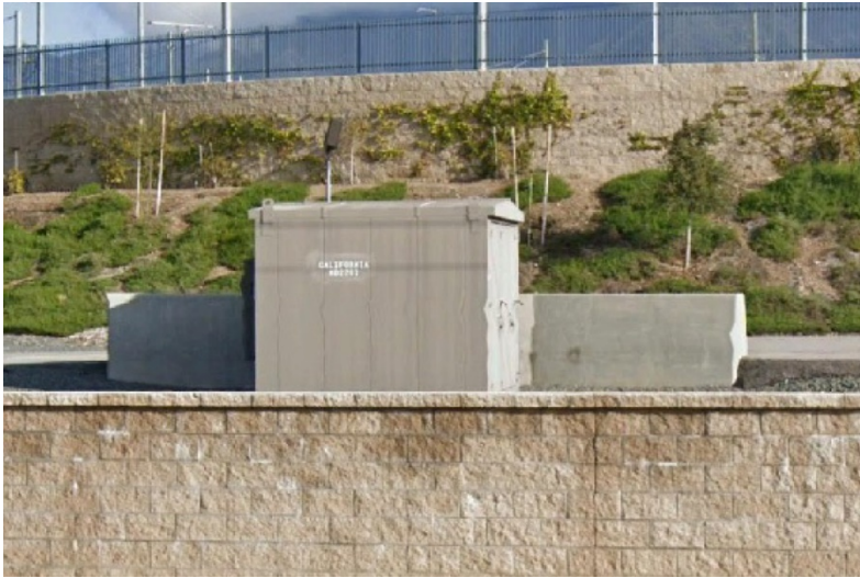
Figure 1-8. Example of Train Control House (Metro L (Gold) Line, Monrovia Station)
