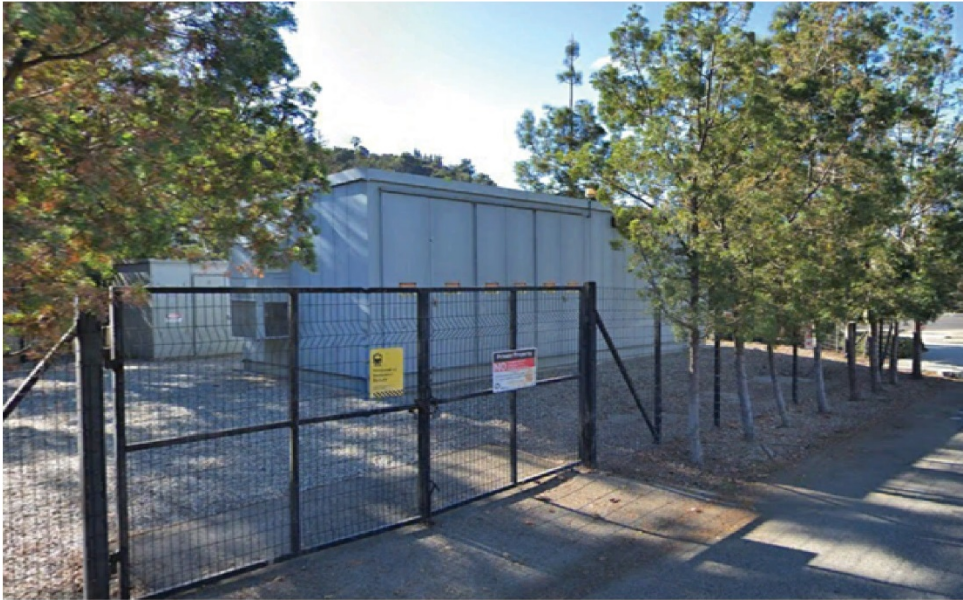
Traction Power Substation Facility on the Metro L Line
