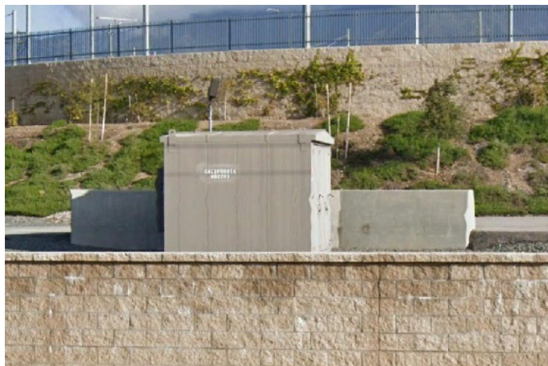
Figure 1-7. Example of Train Control House (Metro L [Gold] Line, Monrovia Station)
