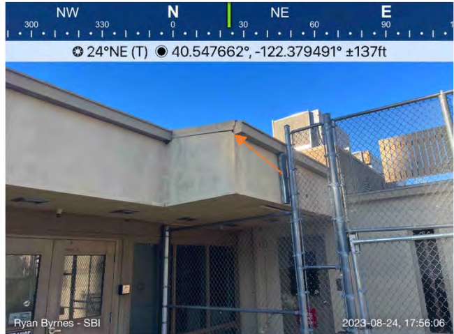
Photo 4. Orange arrow indicating a bat entry and exit point observed on the west side of the Ole Juvenile Justice Center near the western yard.
