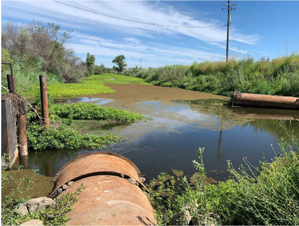
Photograph 1. Tule Canal looking north. Left side of photo is the site of proposed concrete headwall fish barrier. (June 2022)
