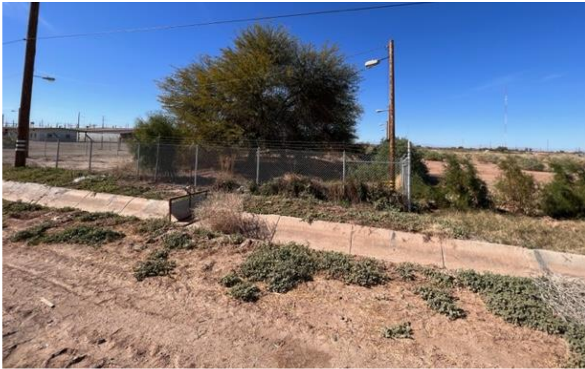
Photo 11: View of concrete lined canal along west side of Dogwood Road (looking west).
