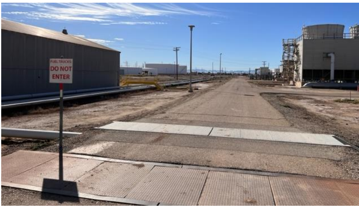
Photo 2: View west from entry at Dogwood Road of internal road to the ECGS Wastewater Facility. Pipeline will be installed in the unpaved area at left of photo.
