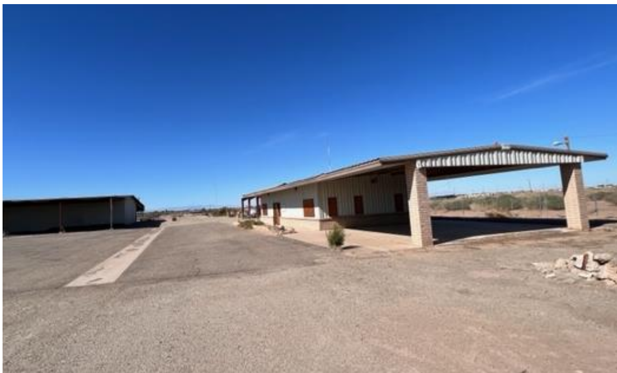
Photo 12: View west from Dogwood Road of existing Bonanza Building and surrounding structures located at the northwest corner of Dogwood Road and Villa Avenue to be demolished to accommodate construction of the 9-acre, three cell evaporation pond.
