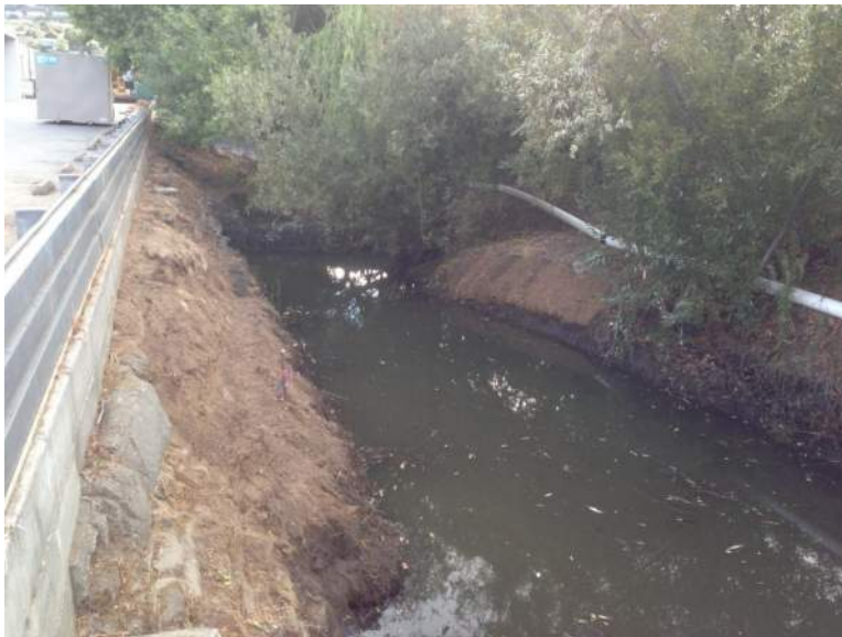
10. Downstream terminus of Project Area showing newly excavated pool that is approximately four feet in depth. This portion of the Project Area is tidally-influenced. A green red willow stake can be seen in the left-center portion of the photograph; the donor tree is located approximately 40 feet upstream. While salinity is a major abiotic stress and limiting factor on the extent of native willow species in brackish water habitats, the presence of red willow and arroyo willow (right side of the photograph) at the high tide limit indicate that these species appear to be acclimated to existing site conditions.
