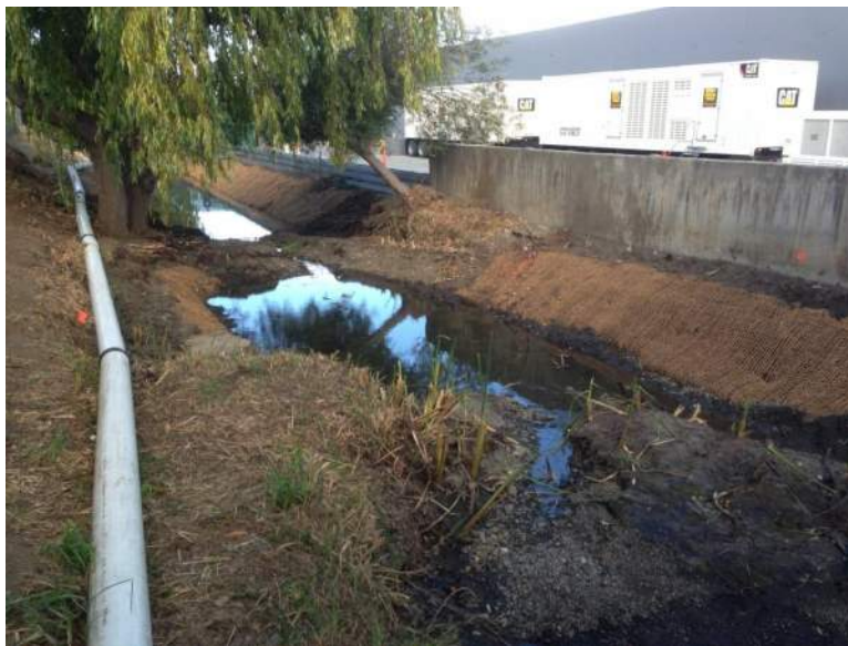
4. Upper reach of Project Area showing post-excavation pool area armored with Coir netting. Red pin flag on the right shows the location for white alder container planting; left pin flag is for western sycamore.
