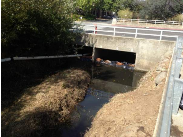
3. Photograph shows downstream coffer dam and by-pass pipe outfall underneath Industrial Road.
