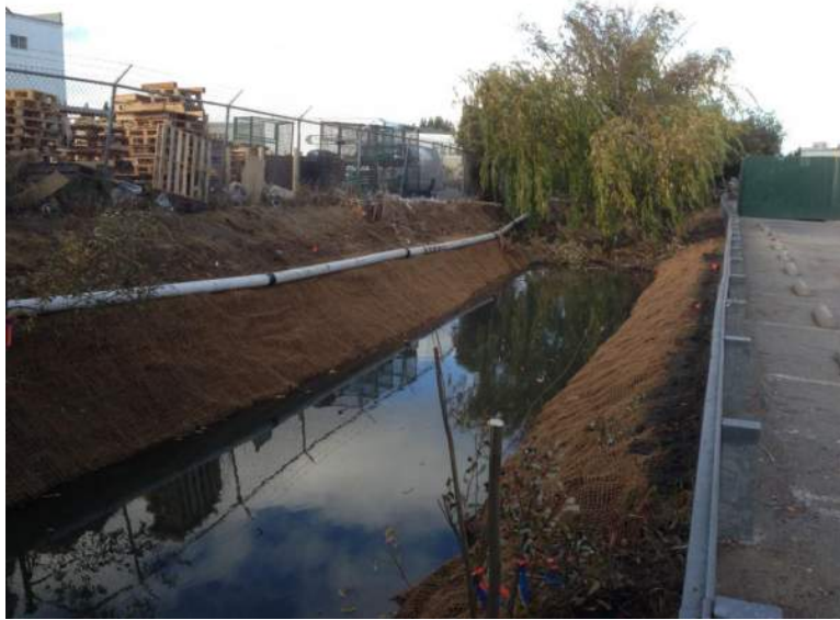
5. Upper reach showing Coir netting and placement of pin flags to mark container planting locations. Blue and orange-flagged green willow stake can be seen in the foreground.
