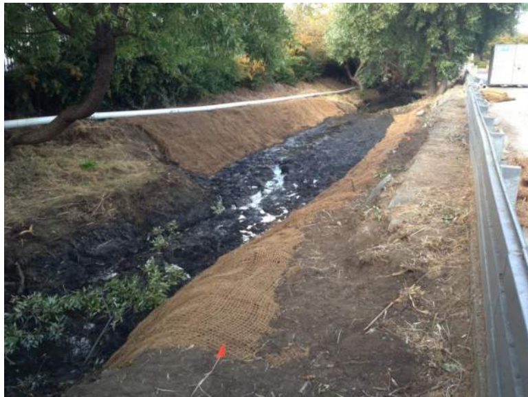
8. Facing downstream, photograph shows lower reach of Project Area showing bank armoring and container planting pin flag locations.
