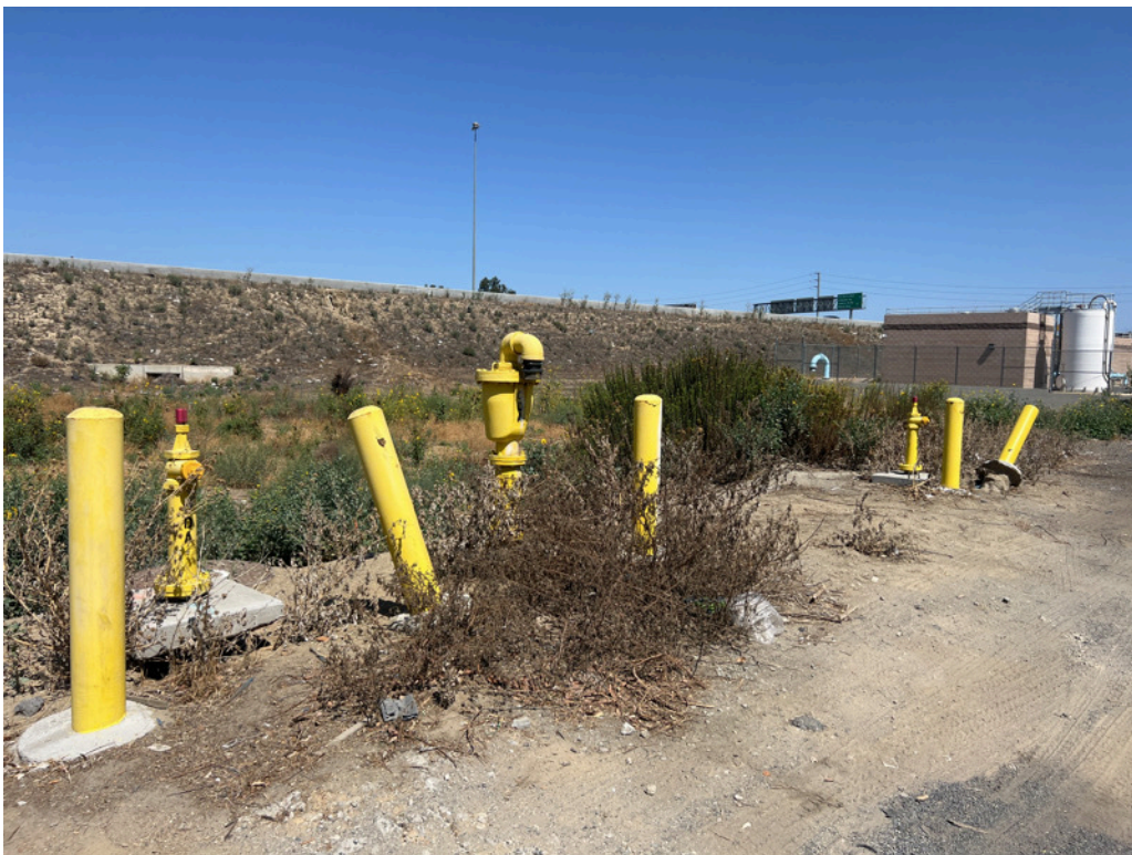
10. Close up of yellow water hydrants at the south subject property boundary
