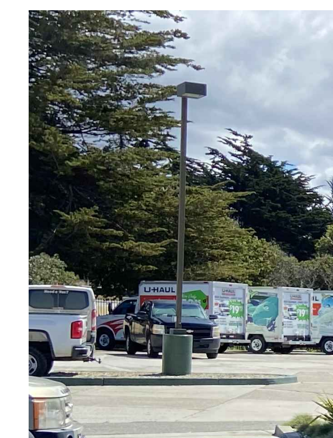
EXISTING POLE LIGHT
