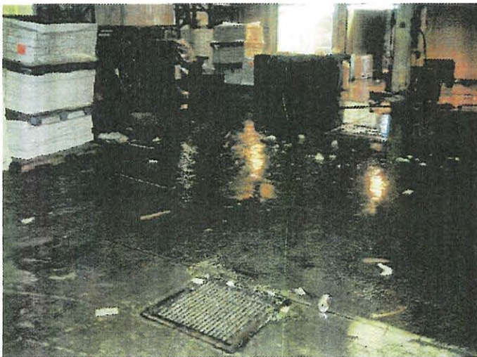
INTERIOR FLOOR DRAIN
