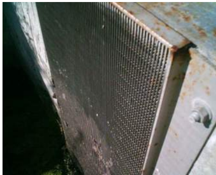
Trash rack with screen
