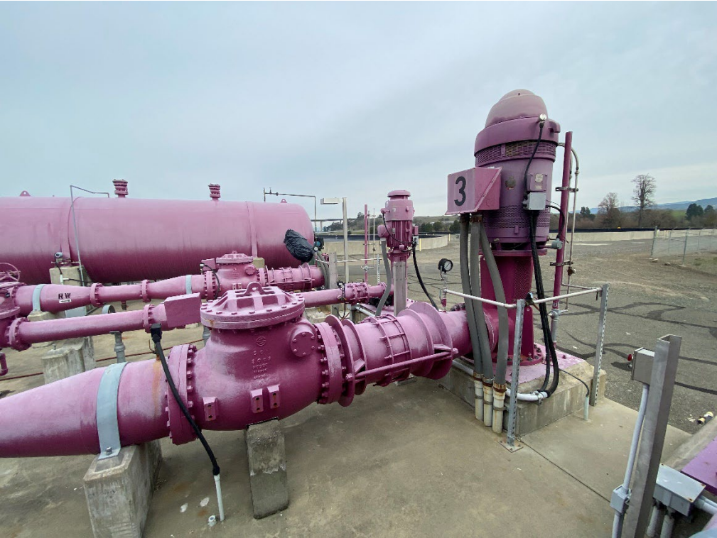
Figure 2-5: Close Up of the SPS
