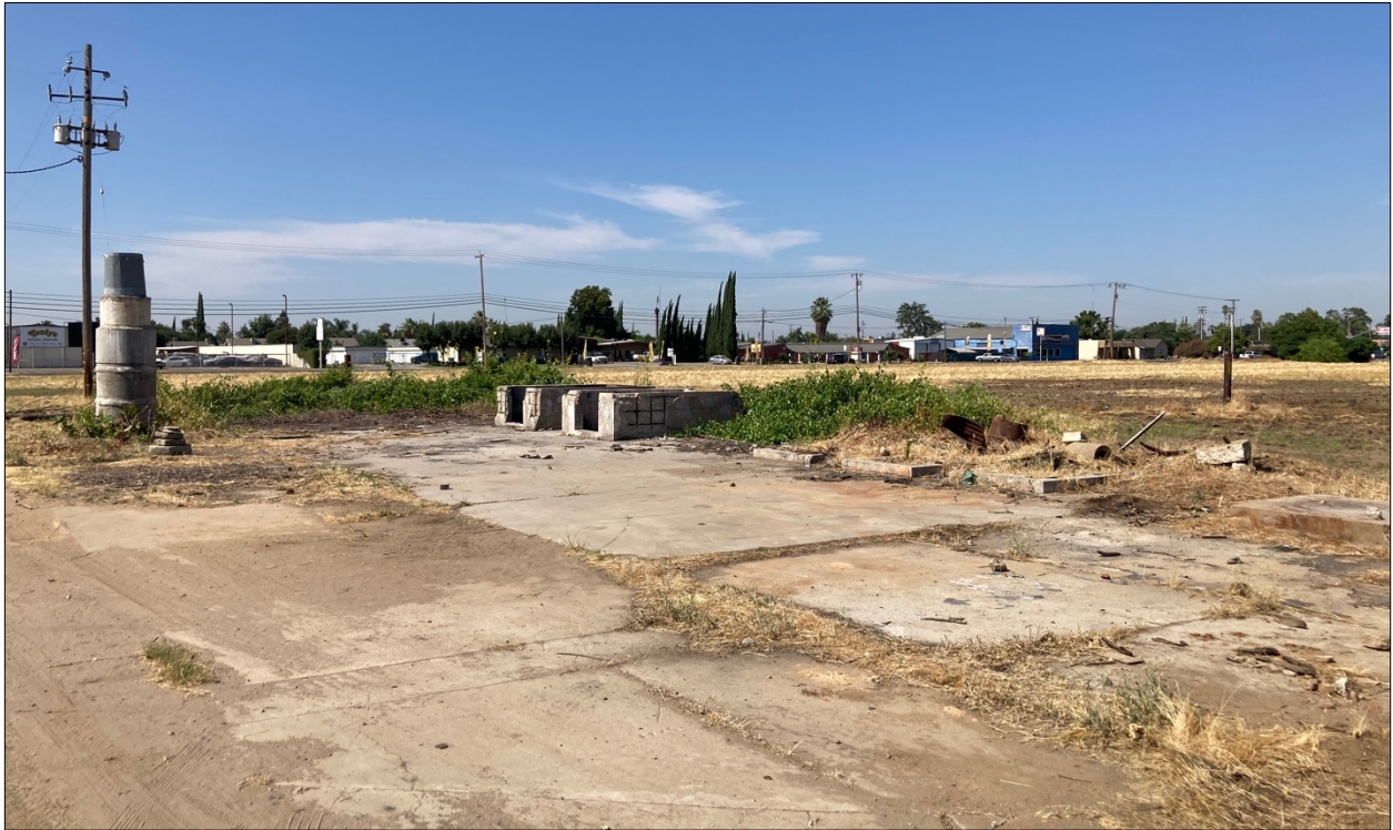
Figure 7. Photograph of the Project site, looking southwest, showing an old concrete foundation.
