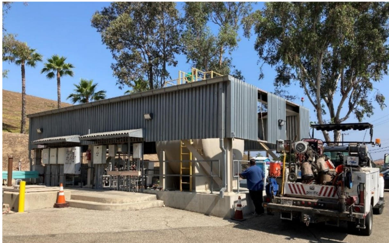
Photograph 3. Sodium Hypochlorite Tank Farm
