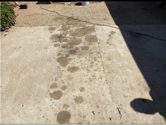
View of oil stains - de minimis observed on rear side of the residential building 26399 Murietta Road
