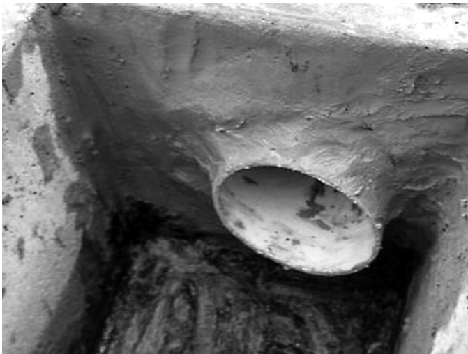
Example of a BAD pipe installation. Protruding past the internal wall of the structure, poor grouting, and wrong position.
