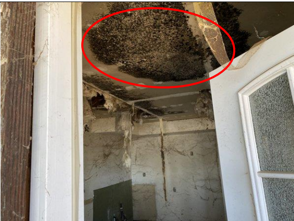
View of mold
