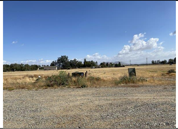
View of pad mount transformer along Elm Street
