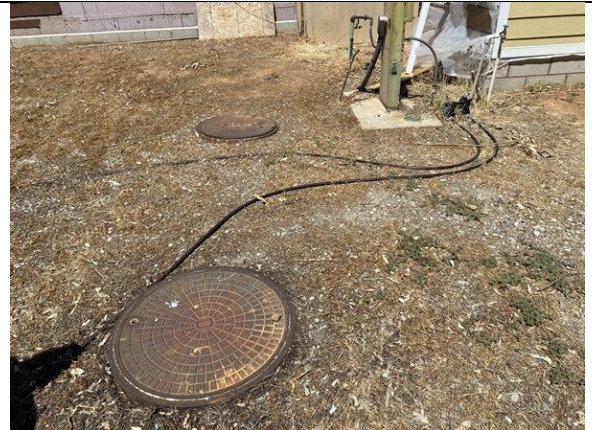
View of septic system located on southside of the Property
