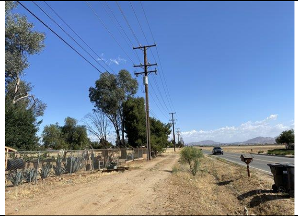
View of pole mount transformer along east side of the Property along Murietta Road
