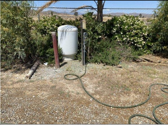
View of water well located on west side of the residential building at 25981 Elm Street
