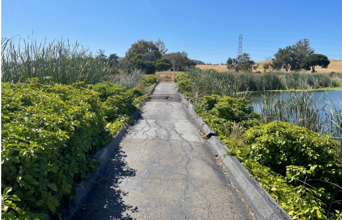
Photo 1. View of Existing City Bridge #25 looking southeast across the top of the existing deteriorated causeway. 1
