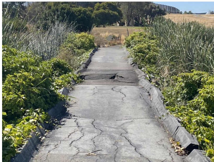
Photo 2. Closeup of existing deterioration Bridge #25.
