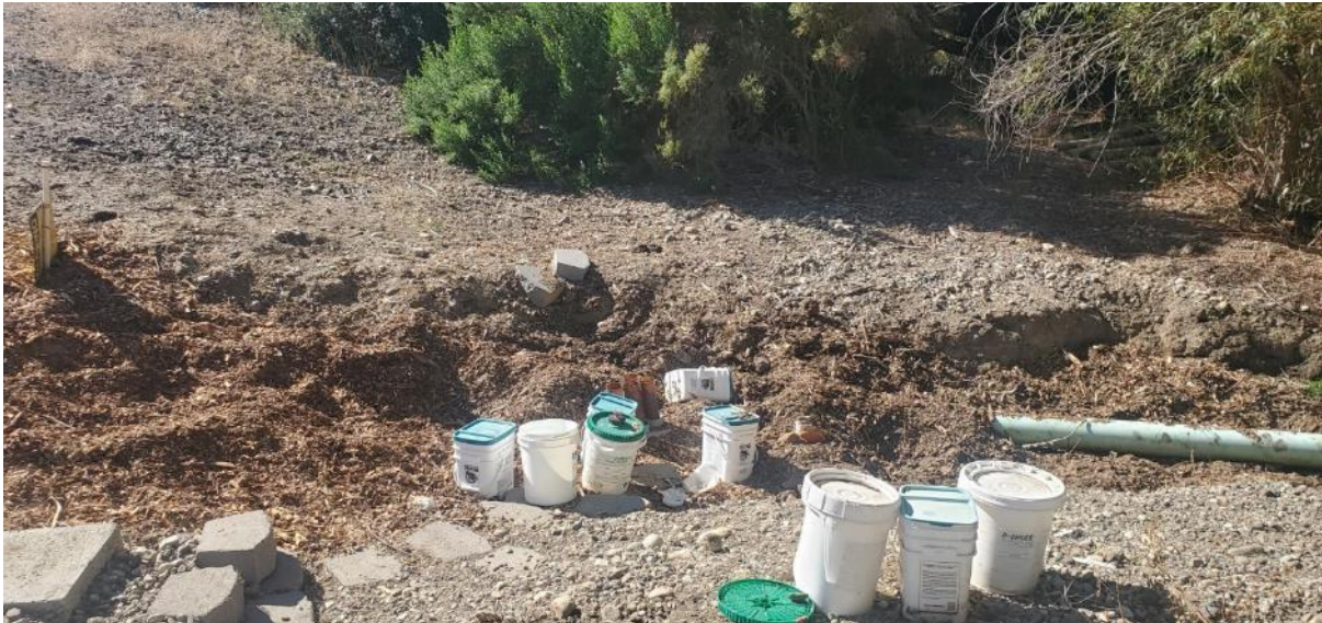
Photograph 4. Photograph of the de-chlorination process replacement location at the spray field, facing west. October 6, 2022.
