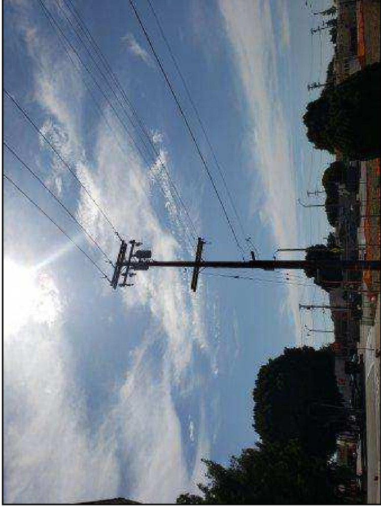
7 : Looking south of the one pole mounted transformer on the eastern portion of the site.
