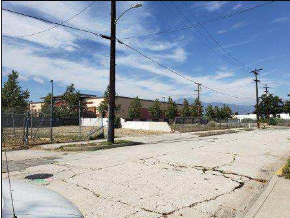
6 : Looking northwest of the three pole-mounted transformers on the western portion of the site.
