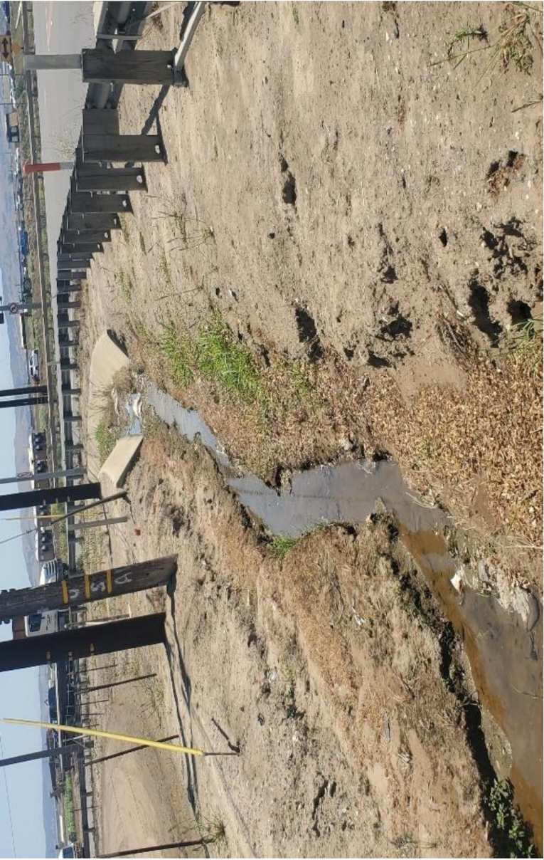
Photograph 1. Photograph of the ditches on the east side of Bonita School Road, facing south. June 28, 2023.
