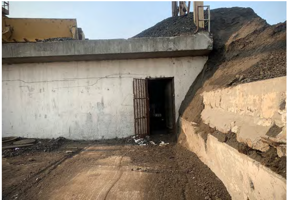
Photograph 8: Looking south at the entrance to the storage room located on the northern end of the concrete platform.
