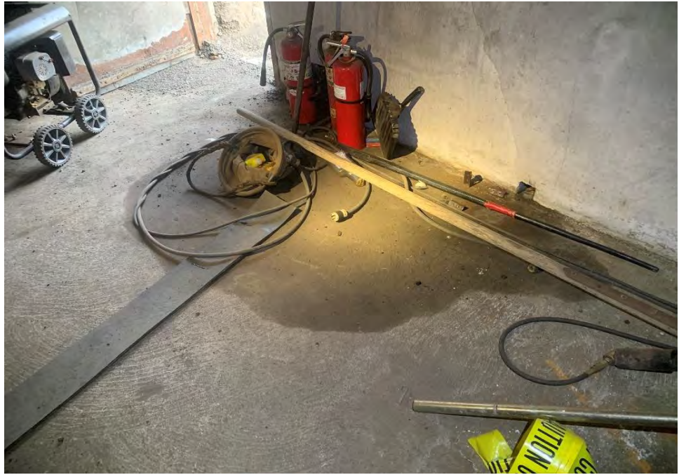
Photograph 9: View of staining on concrete floor inside the entrance of the storage room.
