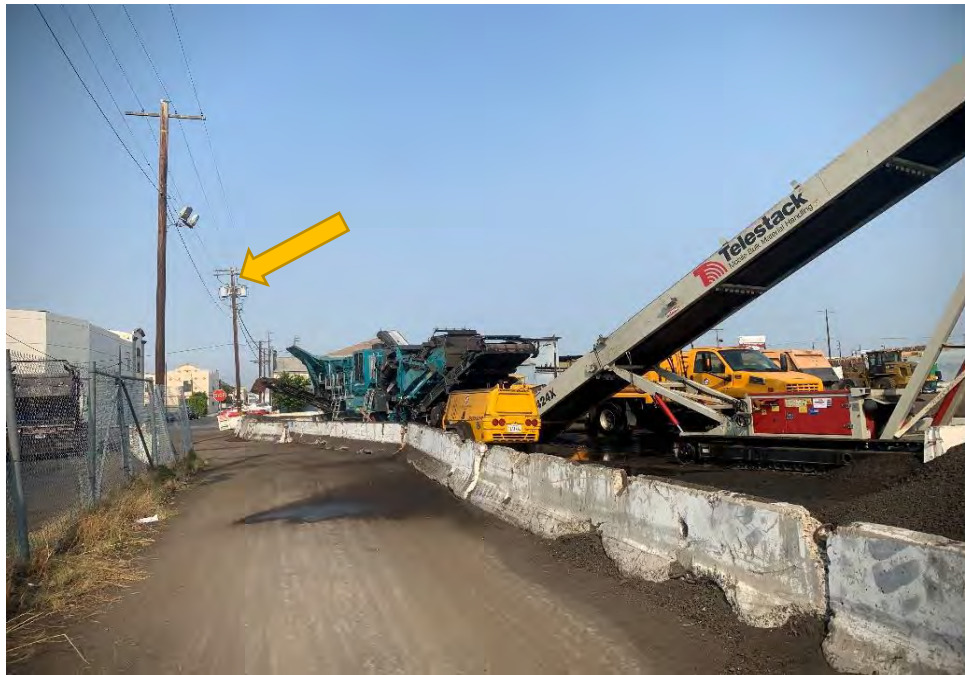
Photograph 1: Looking west along the ramp on the southern boundary of the site, with view of pole-mounted transformer (arrow) at the southwestern corner of the site.
