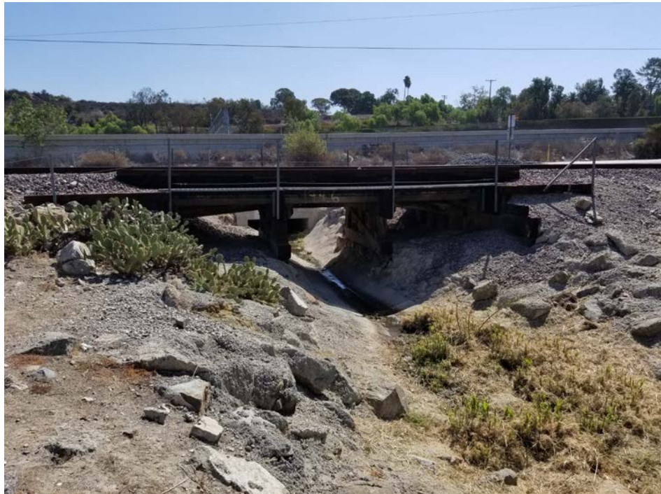
Figure 3. Overview of overpass, associated feature located within Segment 1 of P-19-186804/P-30-176663, view facing east.
