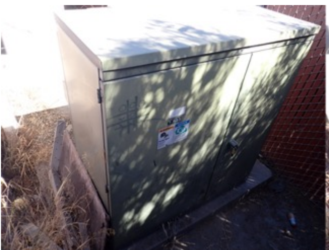
11. View of pad-mounted transformer along northwestern property boundary.
