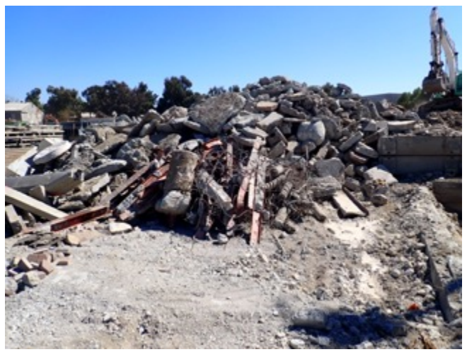
8. View of concrete debris piles prior to crushing, located near center of property.
