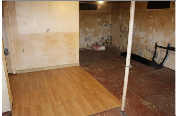
16. Interior view of the subject property featuring the 1271 East Julian Street residential building with a basement space.
