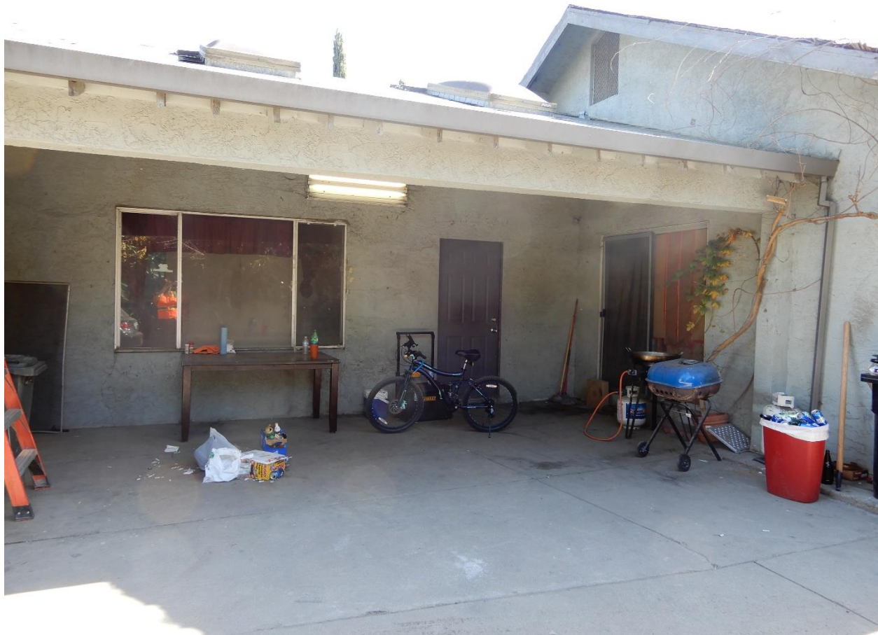
1271 E. Julian Street, detail of recessed bay at west façade, view southeast (ARG, March 2021)
