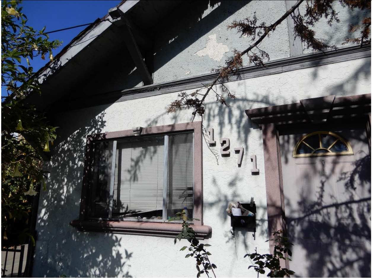
1271 E. Julian Street, detail of west side of primary (south) façade, view north (ARG, March 2021)
