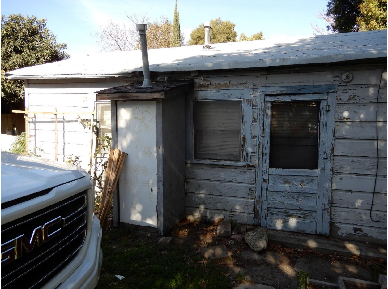
1279 E. Julian Street, one-story residential building, partial view of south façade, view northwest (ARG, March 2021)
