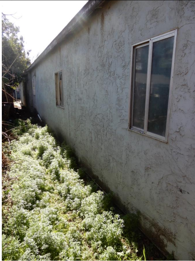
1271 E. Julian Street, partial view of east façade, view south (ARG, March 2021)
