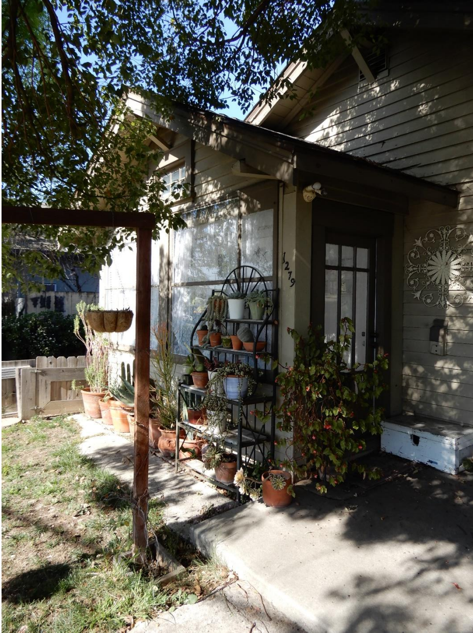
1279 E. Julian Street, detail of entry porch at west side of primary (south) façade, view northwest (ARG, March 2021)
