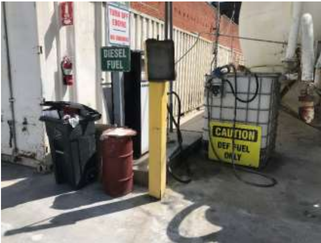
21. Eastern adjoining diesel dispenser.
