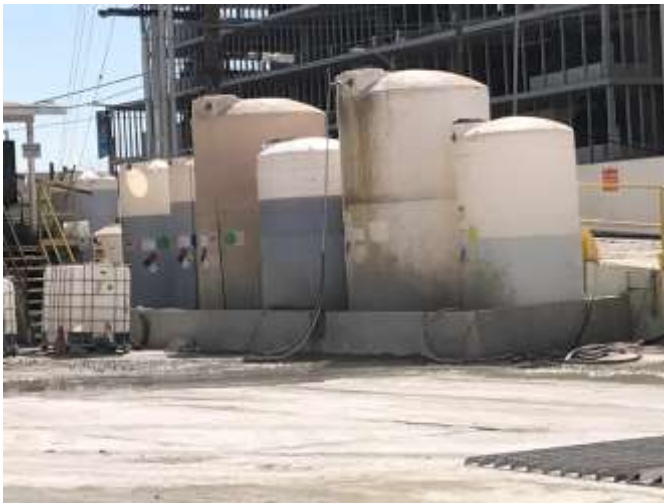
9. View of the ASTs at the mixing tower.
