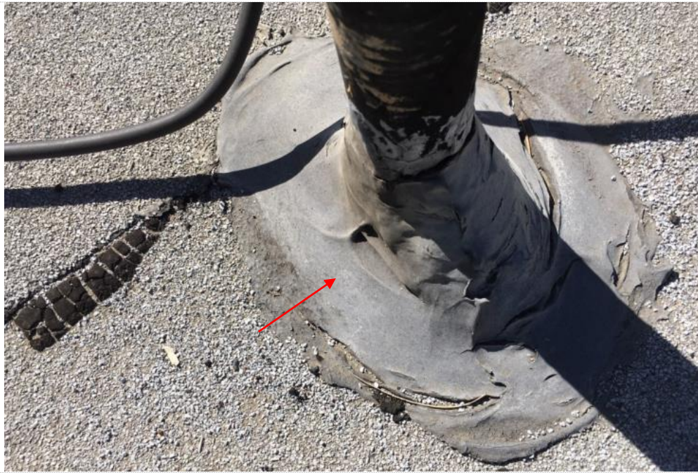
Photo #7: Photo of positive sample group 0610-04 – Gray Roof Penetration Mastic
