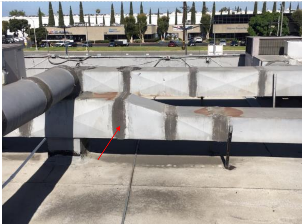
Photo #8: Photo of positive sample group 0610-05 – Gray HVAC Duct Mastic
