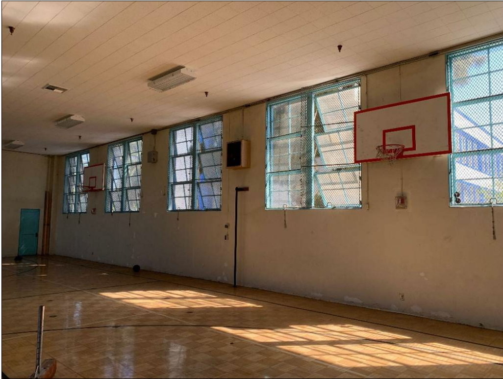
Figure 60. Parquet wood floor and awning-type windows in gymnasium of Physical Education Building.
