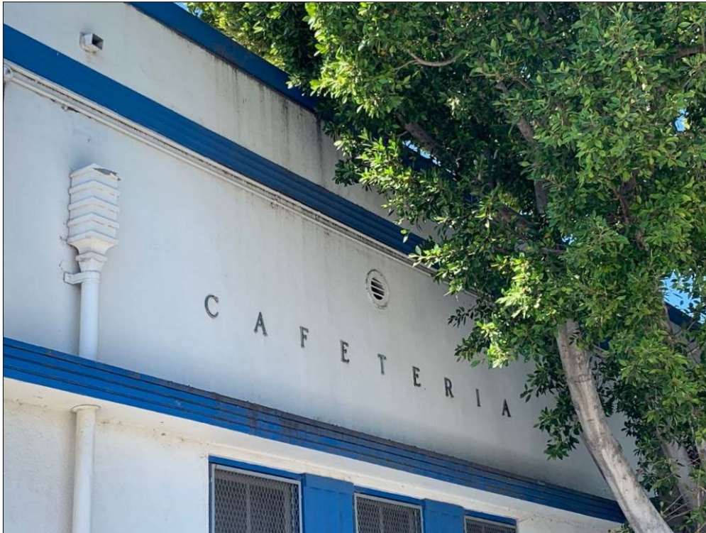
Figure 63. Lettering identifying building, round vent, and square catchment below scupper on Cafeteria.
