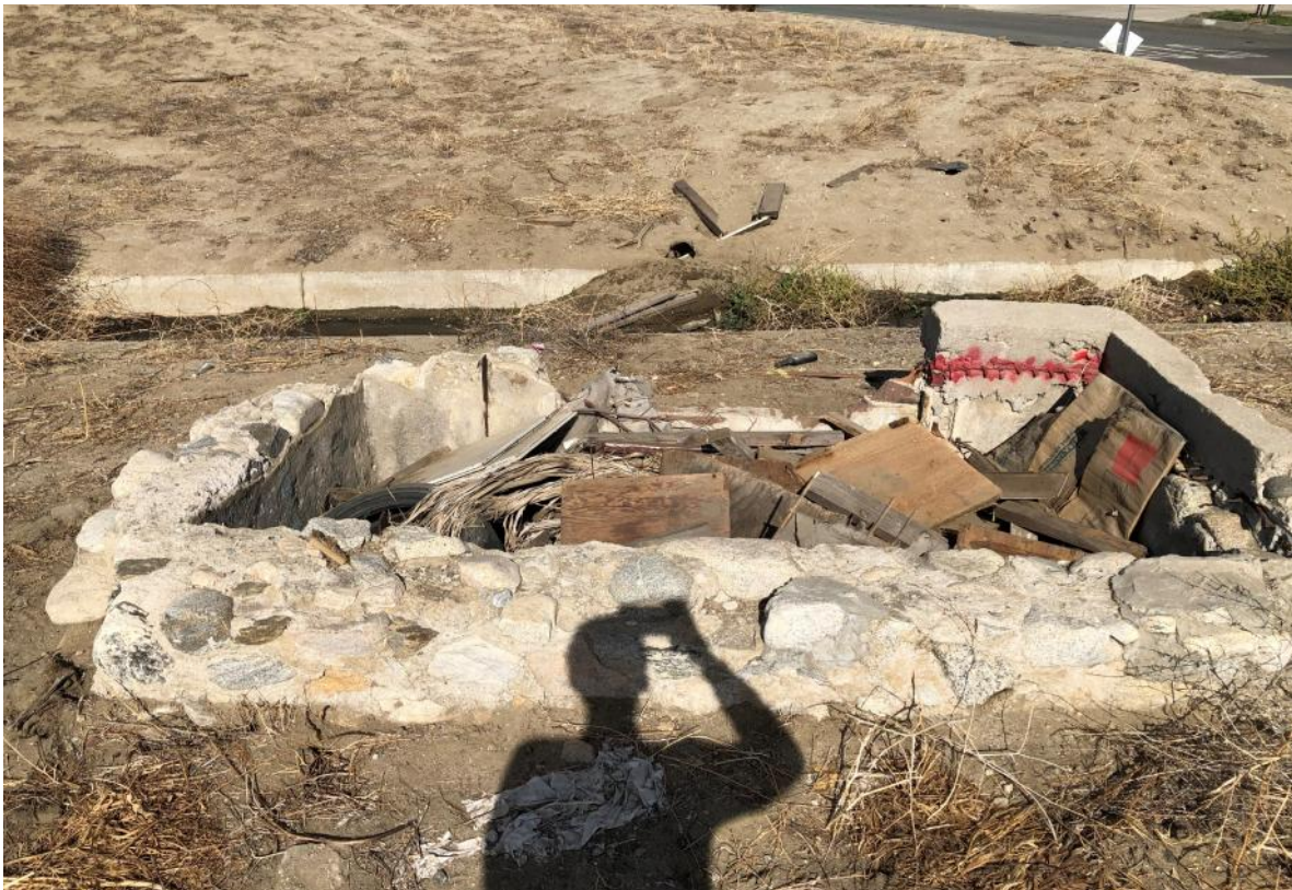
Photograph No. 6: Rectangular-shaped structure in northeast corner of site and U-shaped concrete drainage structure in background trending east-west along center line of future extension of Pennsylvania Avenue
