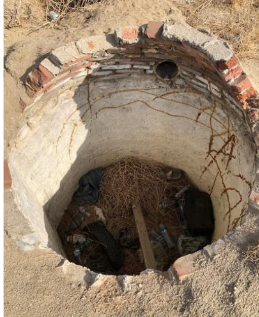
Photograph No. 13: Open cylindrical excavation (shaft) made of brick, concrete and filled with debris in the southwest portion of the site
