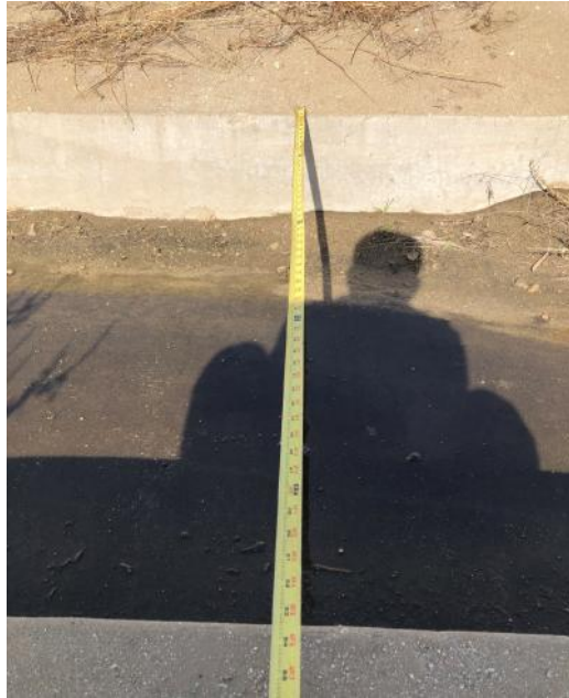
Photograph No. 7: U-shaped concrete structure trending east-west along center line of future extension of Pennsylvania Avenue is about 4.5 feet wide and 12 inches in height
