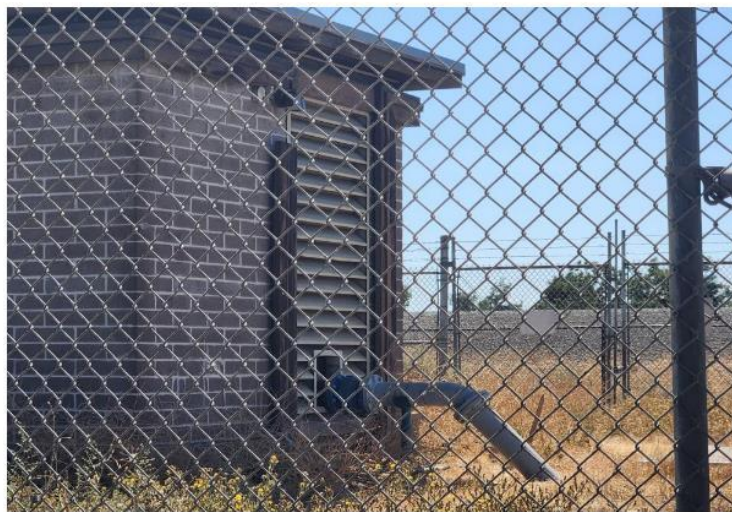
Photograph 3. Pipe leading from well house facing south.
