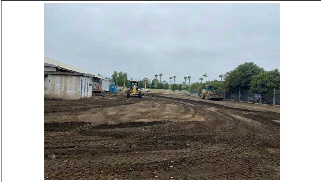
View of site preparation activities from east side of AOC5 facing west (9/2/21).
