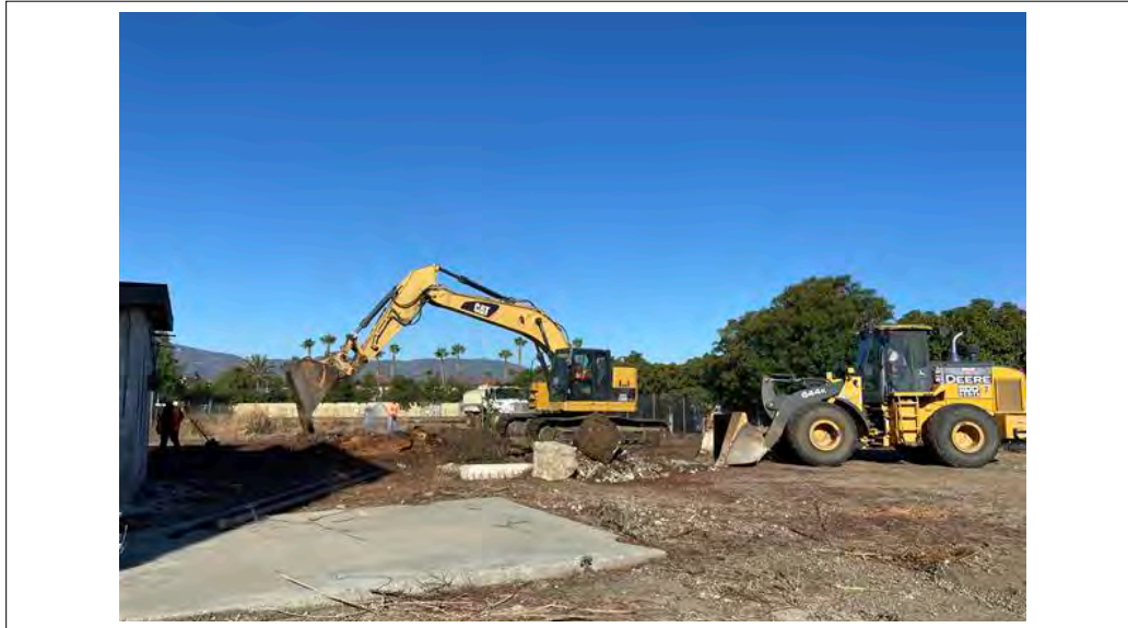
View from stabilized construction entrance at southeast corner of AOC5 facing west. View of breaking/removal of concrete (8/3/21).
