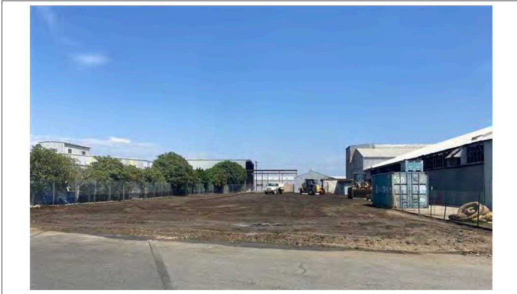
View from west side of AOC1. View of moisture conditioned soil up to the edge of the current asphalt pavement. (8/31/21)
