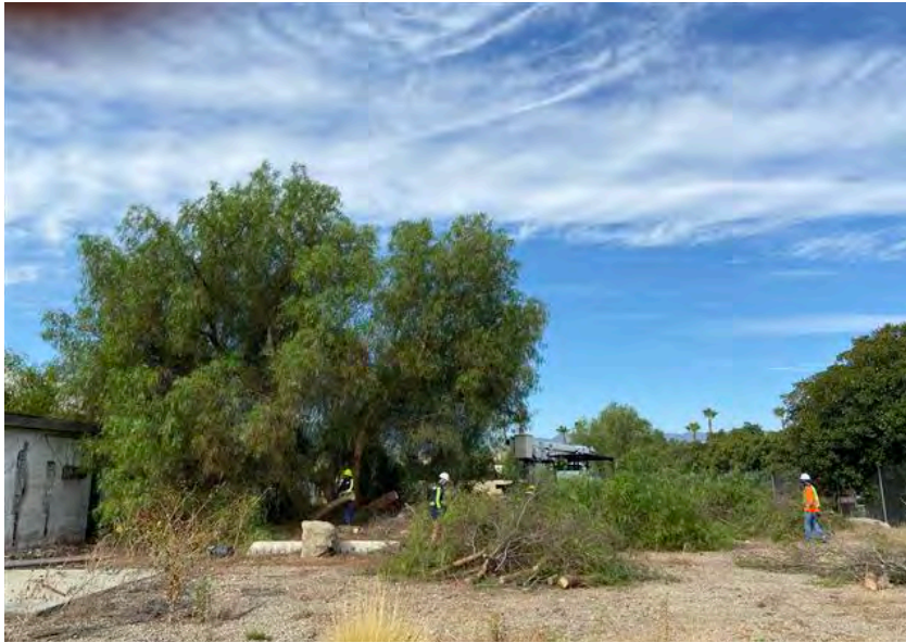
View of AOC1/AOC5 facing west from east side of AOC5 during tree removal (7/30/21).
