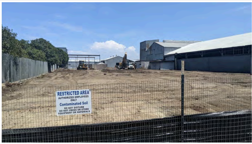
View from AOC1 west boundary after rail lines and ties have been removed (8/10/21).
