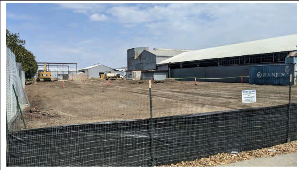
View from AOC1 northwest corner of beginning of hot spot excavation activities (8/11/21).
