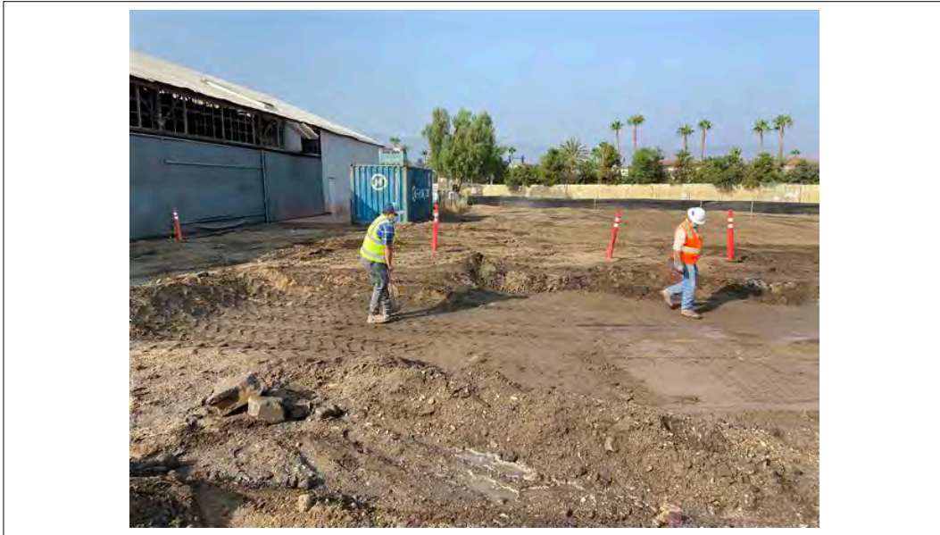
View facing west from AOC1/AOC5. View of Geotech subcontractor collecting data on the backfill of the former septic tank excavation. (8/24/21)
