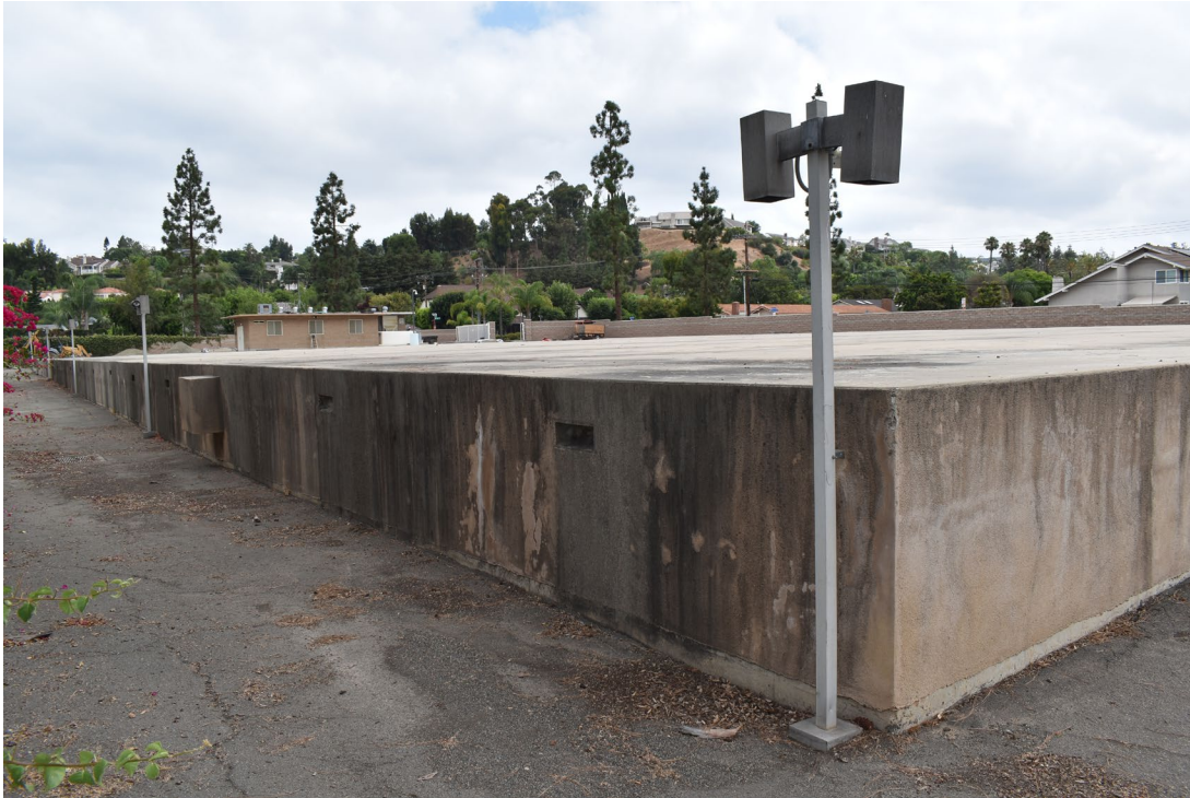
Photograph 2: Reservoir covered with reinforced concrete, camera facing northwest August 11, 2023, Photo taken by Tetra Tech Inc.
