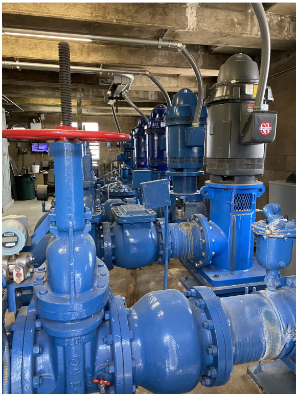
Photograph 5: Interior, pump station, camera facing northeast, August 11, 2023, photo taken by Tetra Tech, Inc.
