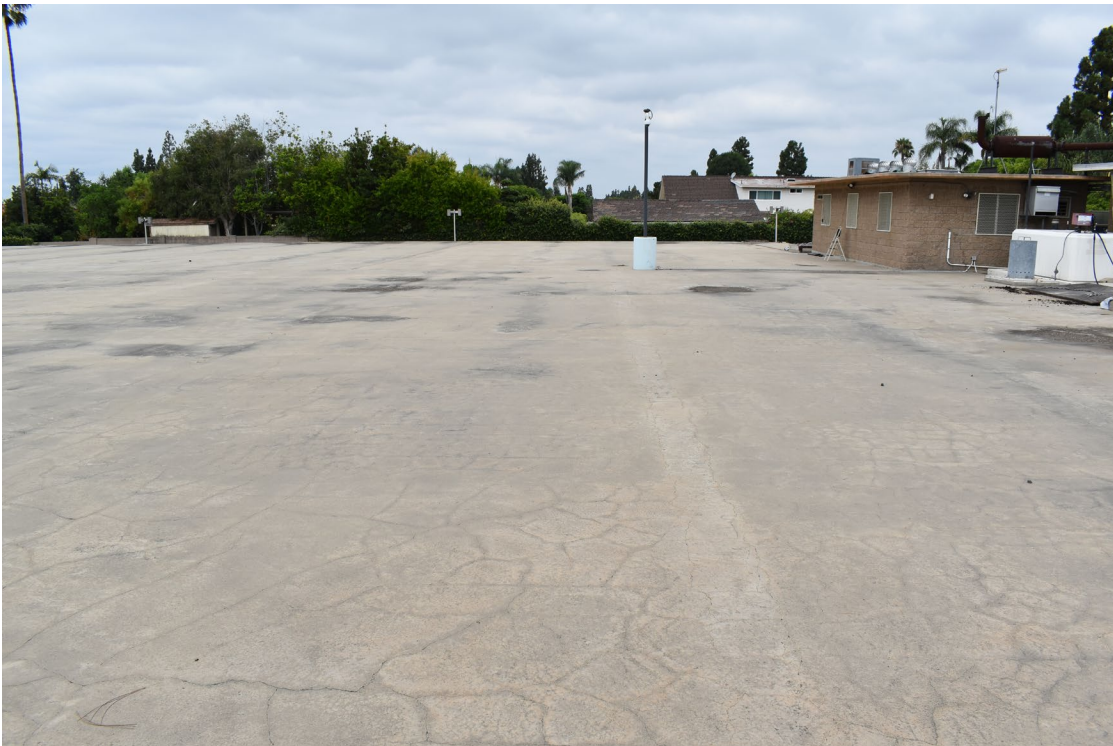
Photograph 3: Reservoir and pump station, camera facing south, August 11, 2023, photo taken by Tetra Tech, Inc.
